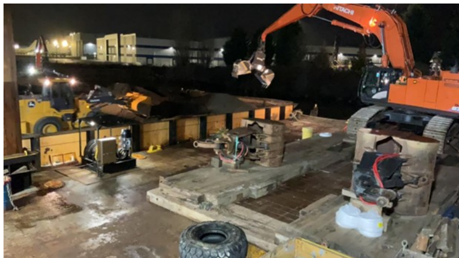
Backfilling must be done during high tides and requires working before sunrise (Photo credit: Geosyntec, week of February 10, 2025).
