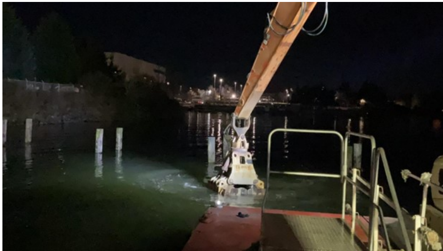
Backfill is carefully placed beneath the water surface (Photo credit: Geosyntec, week of February 10, 2025).
