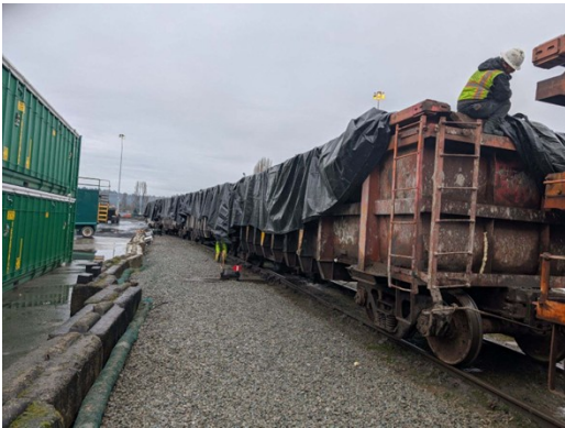
Preparing rail cars for lined and covered transport of dredged material to the landfill. (Photo credit: Geosyntec)
