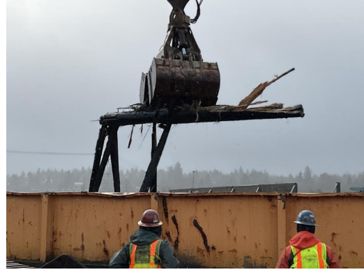
Dredging at SMA 9 removes debris to enable contaminated sediment removal. (Photo credit: Geosyntec)
