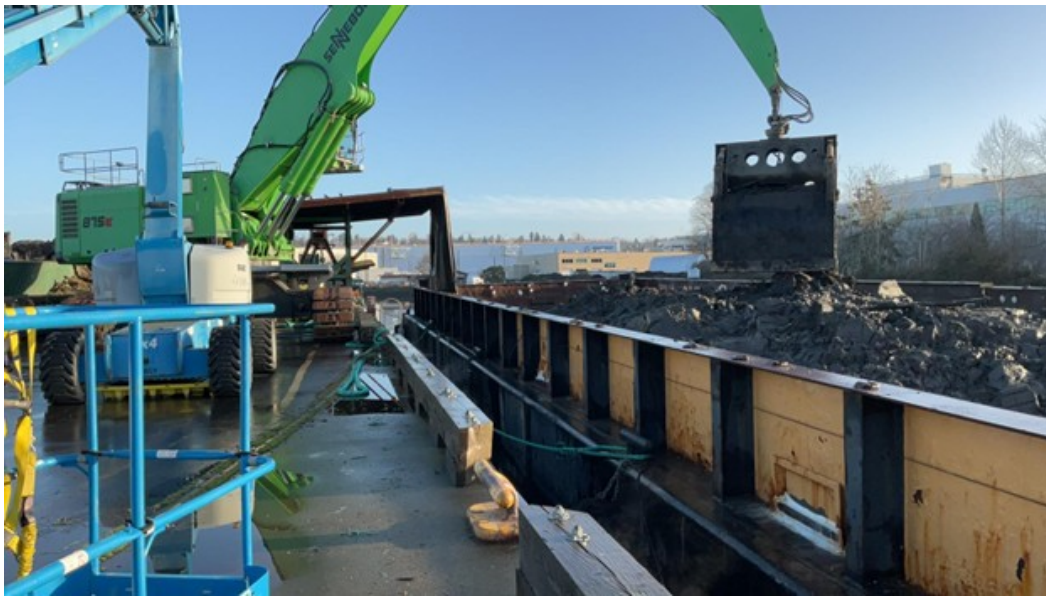
A barge moves material at the transload facility for loading onto rail cars. (Photo credit: Geosyntec)
