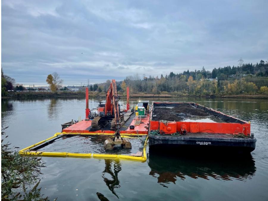
Excavator removes contaminated sediment from the river bottom to place in barge. (Photo credit: Boeing)
