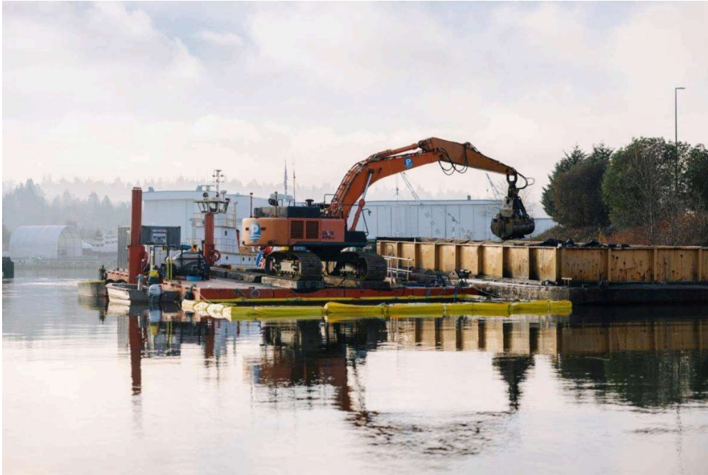
On December 5, an excavator removes contaminated sediment from the river bottom to place in barge. (Photo credit: King County)
