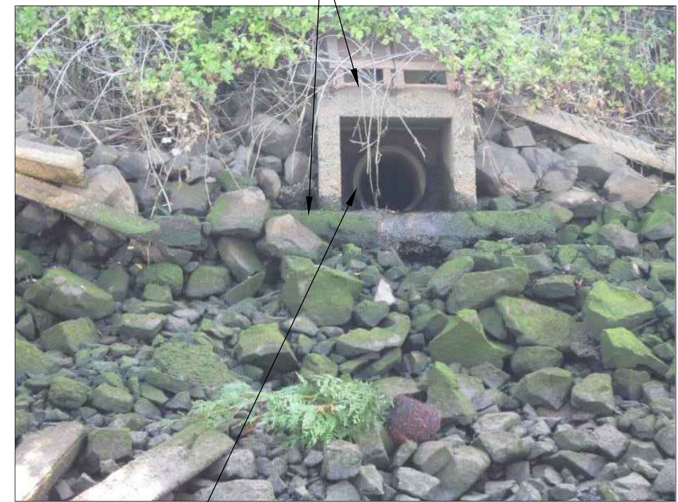
PHOTO 2 SCALE: NONE OUTFALL 2073 18" DIA CONCRETE PIPE (5) 3-SIDED CONCRETE BOX AND CONC SPLASH PAD TO REMAIN IN PLACE. LOCAL BANK PROTECTION TO BE ADJUSTED AS REQD TO INSTALL ENERGY DISSIPATION STRUCTURE (5) (6)
