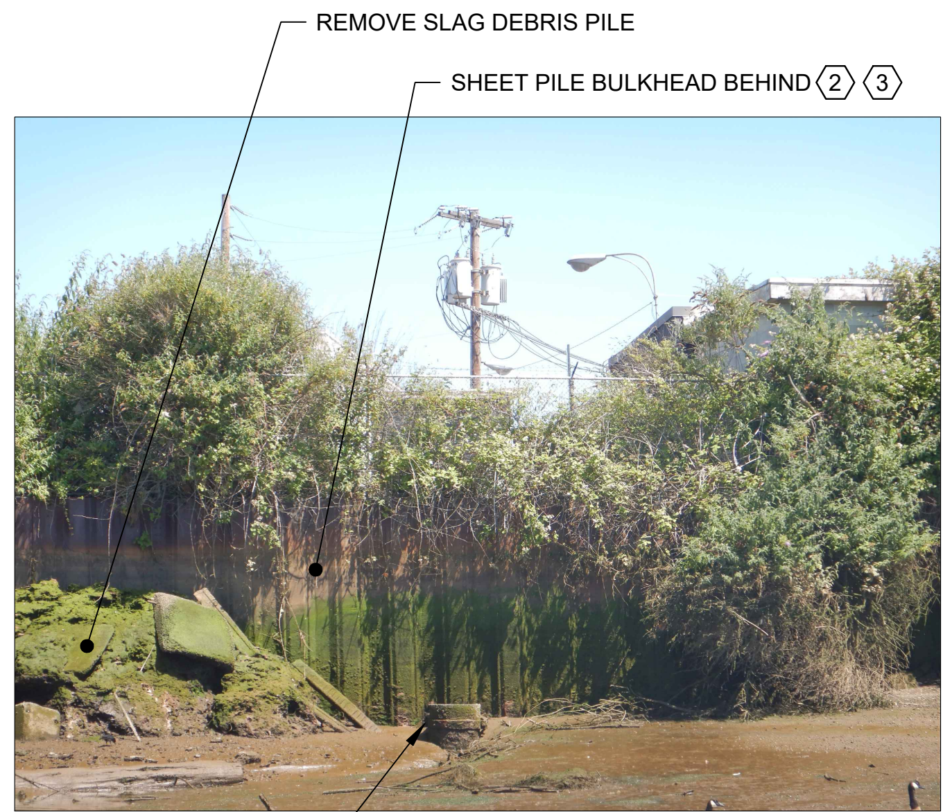
PHOTO 1 SCALE: NONE OUTFALL 2075 32" DIA STEEL RISER (4) OUTFALL 2075 REMOVE SLAG DEBRIS PILE SHEET PILE BULKHEAD BEHIND (2) (3)
