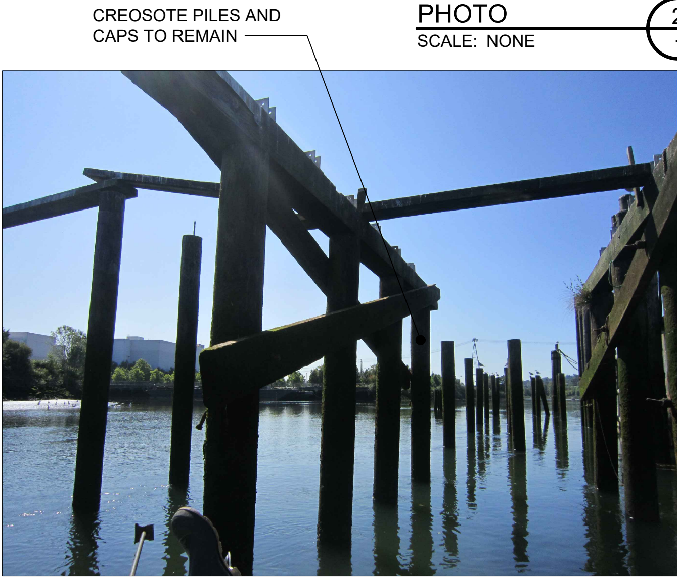
DILAPIDATED L-SHAPED PIER BENT PHOTO SCALE: NONE
