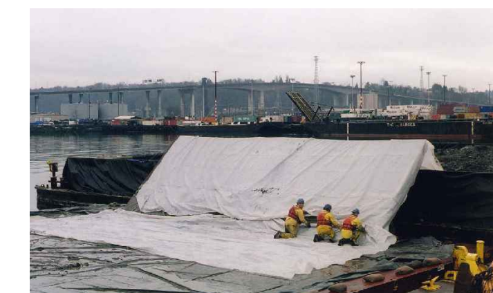
PHOTO 2: EXAMPLE OF OFFLOADING OPERATIONAL CONTROLS
