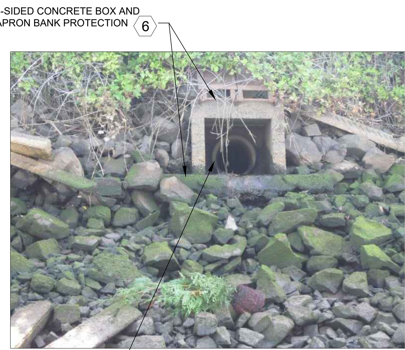
OUTFALL 2073 18" DIA CONCRETE PIPE, IF OUTFALL IS WITHIN DREDGE PRISM, REMOVE EXISTING RIPRAP AS REQUIRED, AND SEE NOTE (6) PHOTO SCALE: NONE (2)
