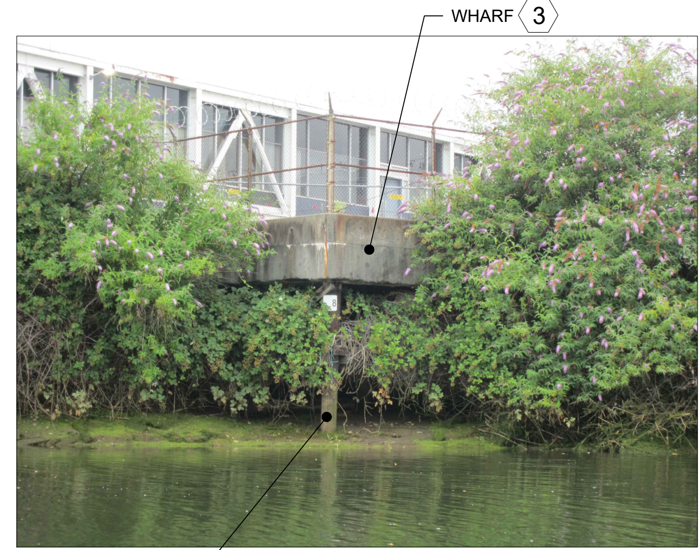
WHARF 3 CREOSOTE PILE TO BE PROTECTED 4 SOUTH WHARF PHOTO SCALE: NONE 1 S-106
