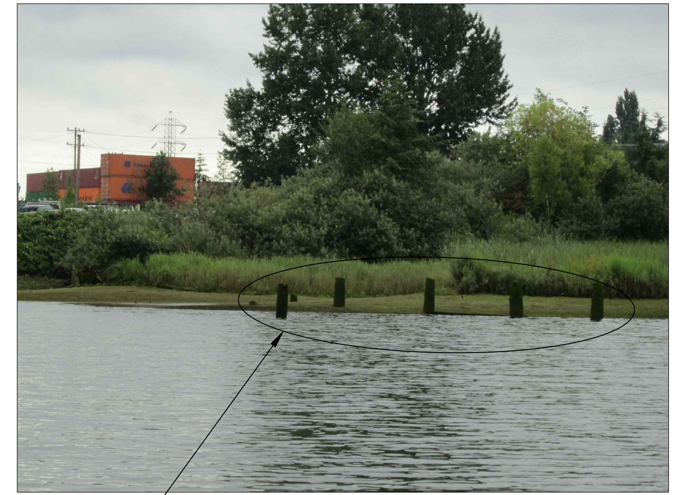
(7) TIMBER PILES TO BE REMOVED. NO REPLACEMENT SINGLE TIMBER PILE FIELD PHOTO SCALE: NONE 2 S-106
