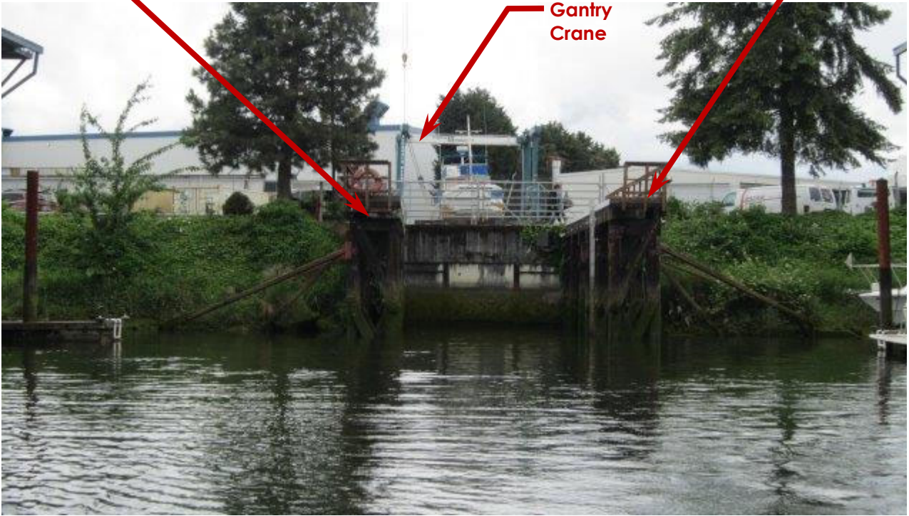
Photo ST14-01: Boat Lift (Looking West)
