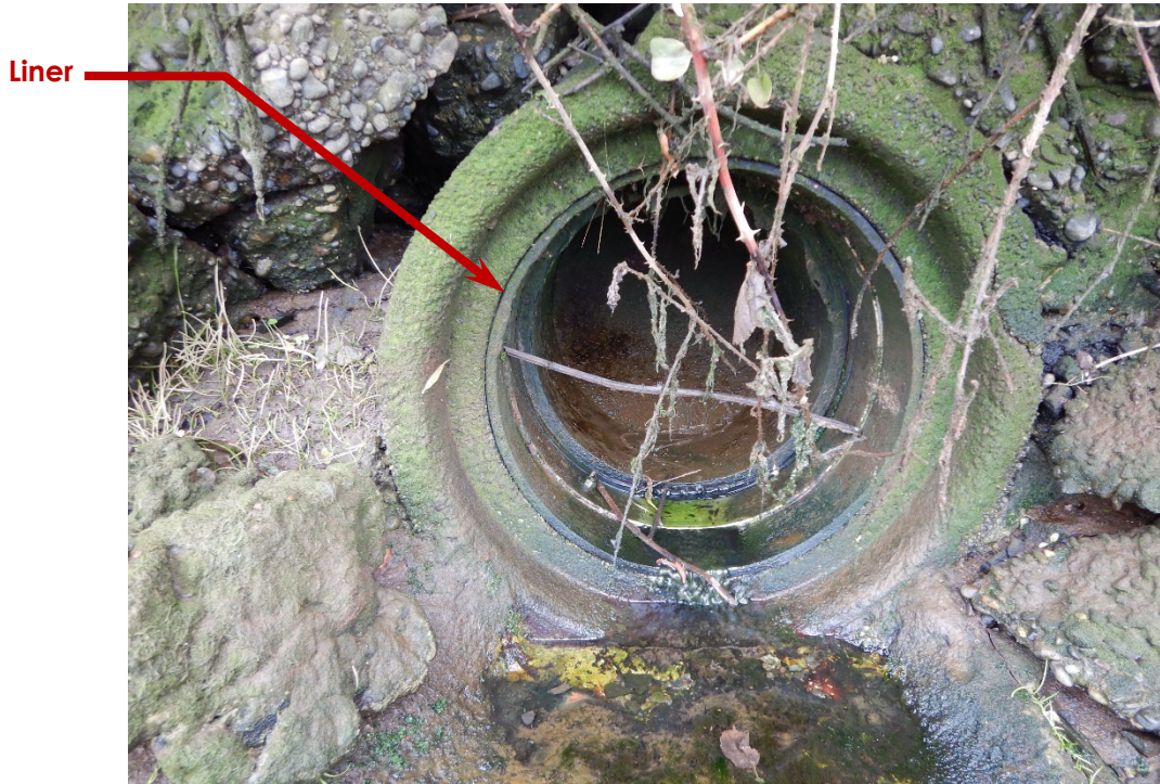
Photo 2093-03: Outfall Close Up
