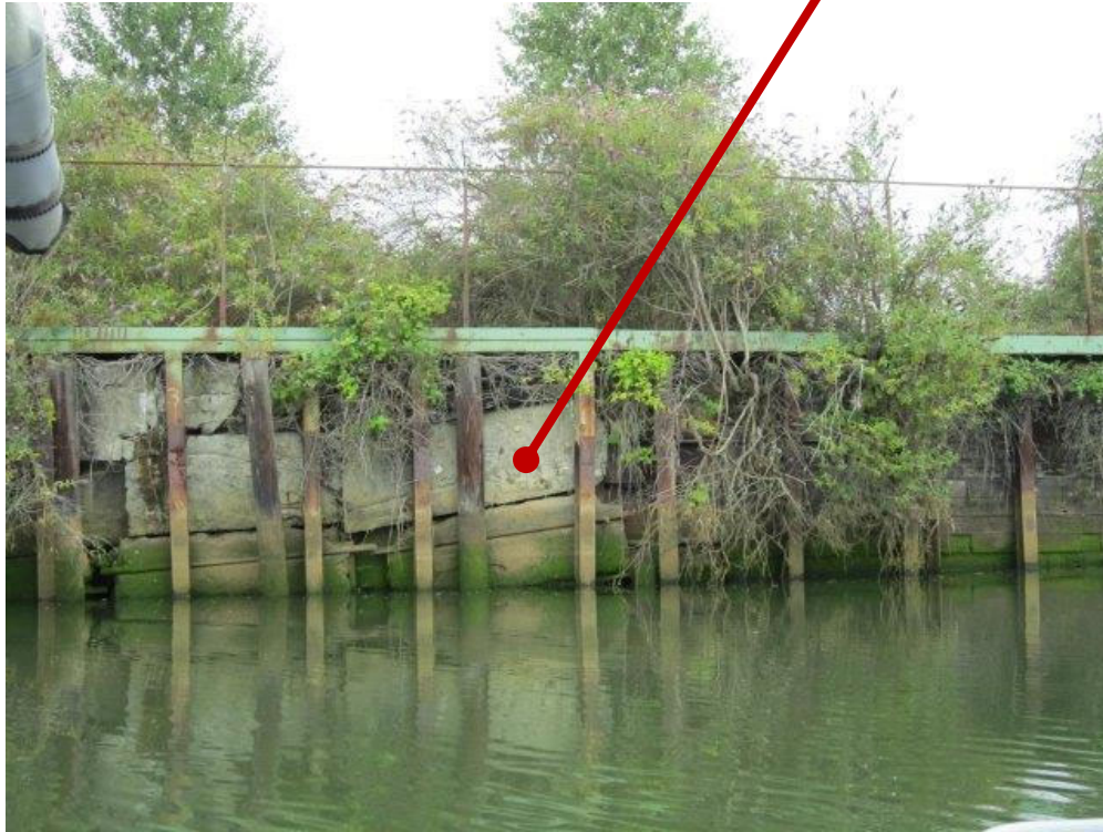
Photo ST03-13: H-Piles with Concrete Panel Rubbles
