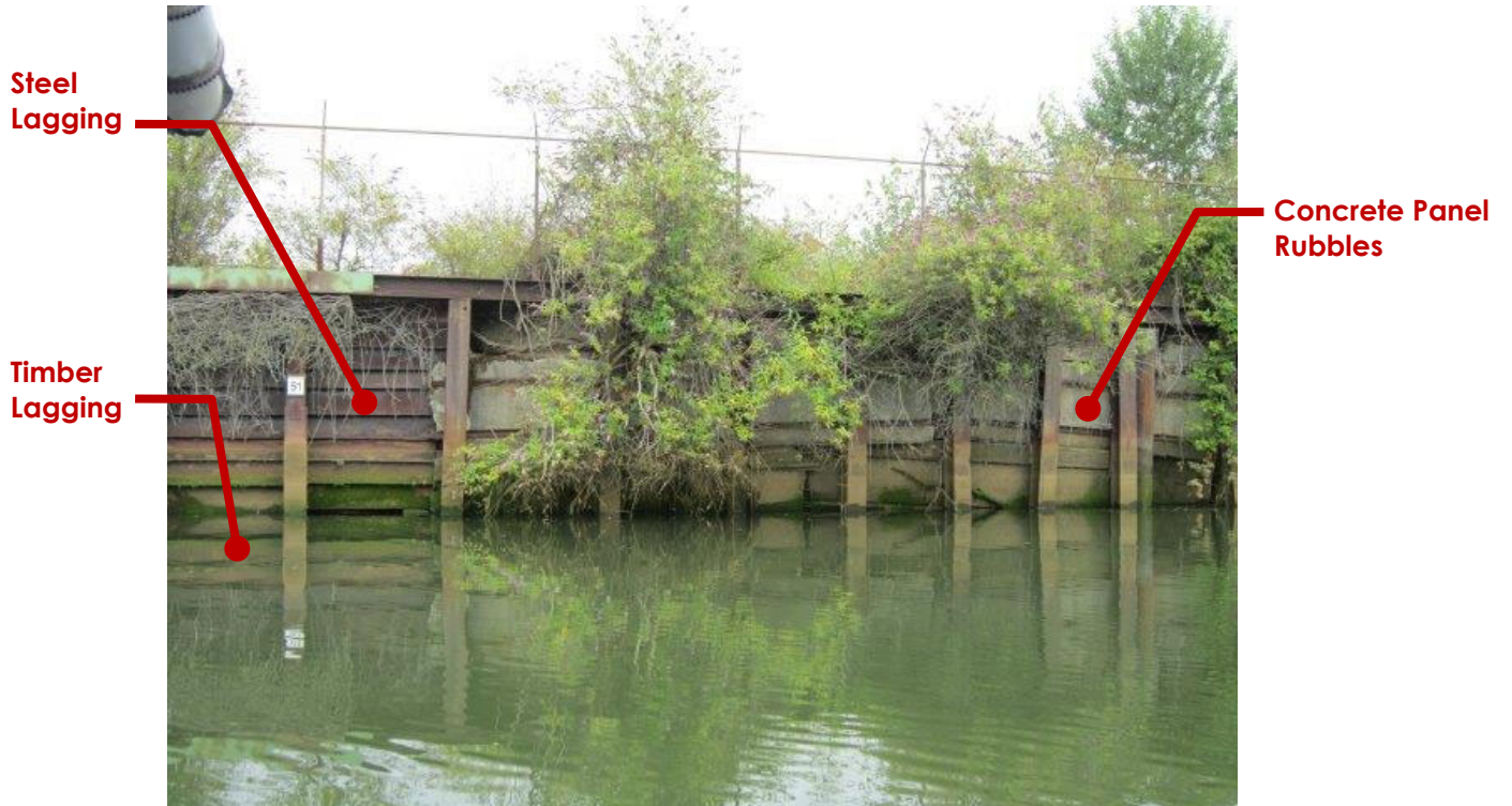
Photo ST03-10: H-Piles with Concrete Panel Rubbles
