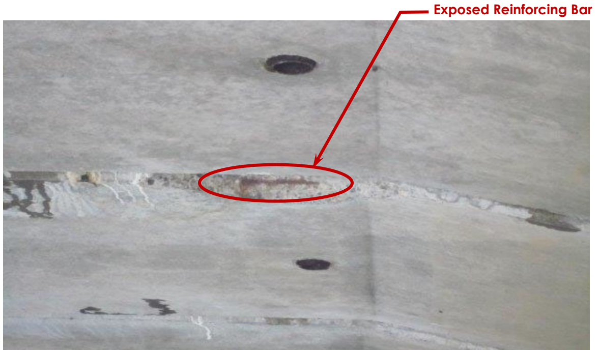
Photo ST05-07: Close Up of Exposed Reinforcing Bar
