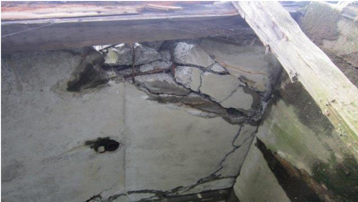
Photo ST05-13: Pier 2, Close Up of West Corner of 1 st Deck Panel
