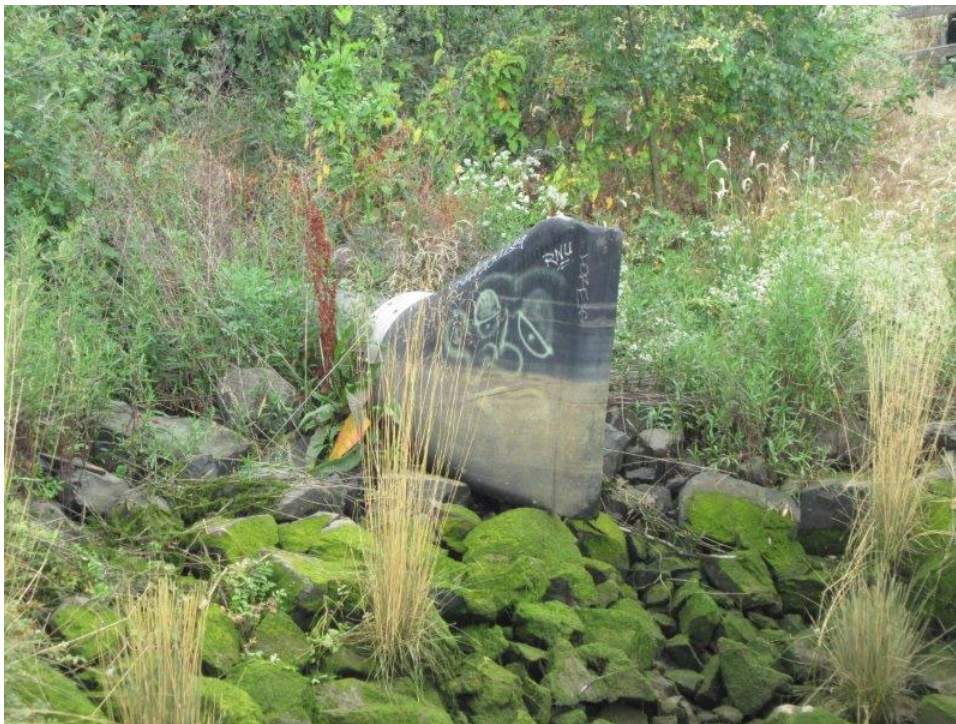
Photo 2215-03: Outfall Close Up
