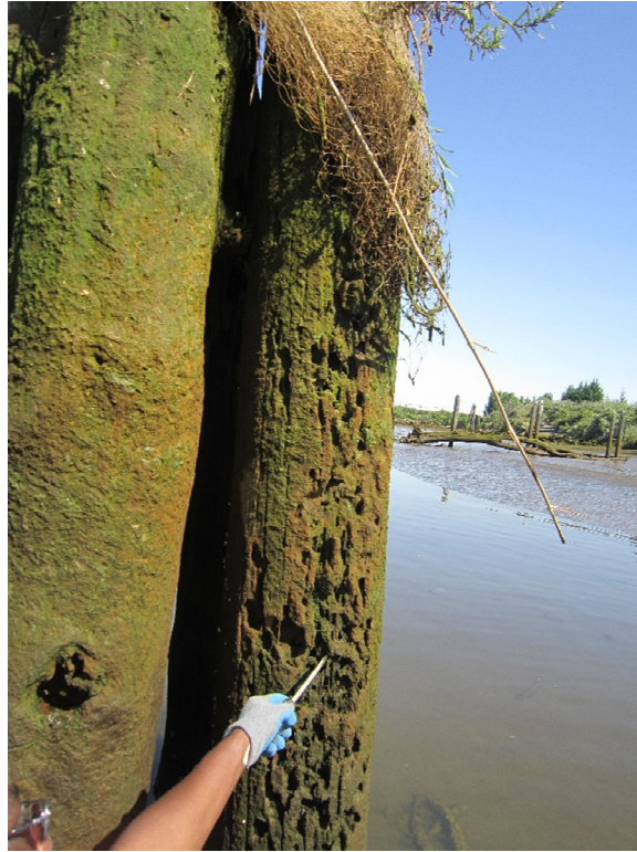
Photo ST04-07: Closeup of Pile Damage
