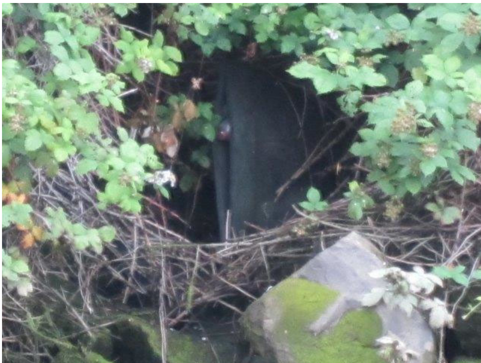
Photo Ditch #2-02: Enlarged Outfall Valve
