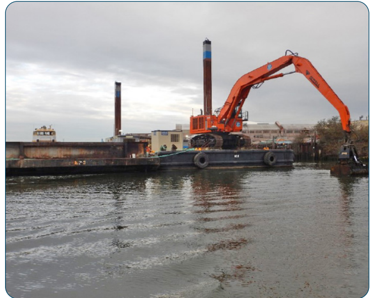
Contractors using a barge-mounted excavator to place study material in the Lower Duwamish Waterway
