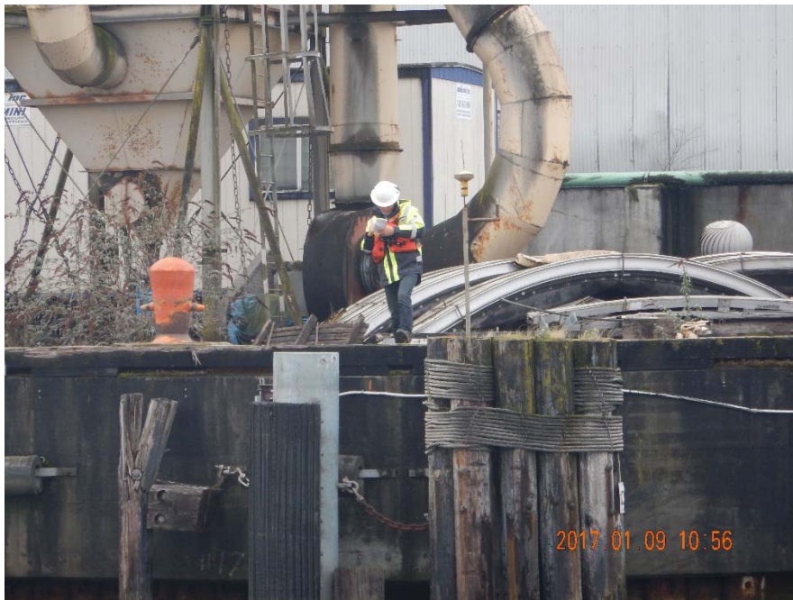
Photo 1-B: Terrasond representative establishing RTK GPS base station at Lafarge dock prior to placement activities at the Sub-tidal plot.
