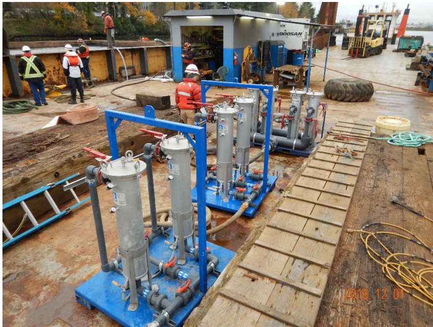
Photo 2-A: The bag filter system used for barge water filtration. The four furthest filters had 25 micron bag filters initially but were replaced with 1 micron filters after a turbidity plume was observed during barge pumping.
