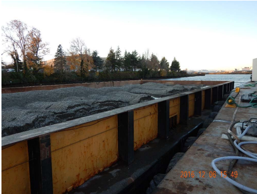
Photo 2-A: KP-3 material barge arrives on-site with Gravelly Sand. The excavator knocked down the wind rows prior to soaking.
