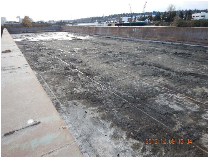
Photo 1-B: KP-2 material barge after all of the Gravelly Sand + AC was placed.
