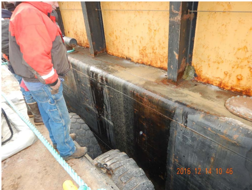
Photo 1-B: Leak observed mid-barge after the material at the base of the bin wall was removed.
