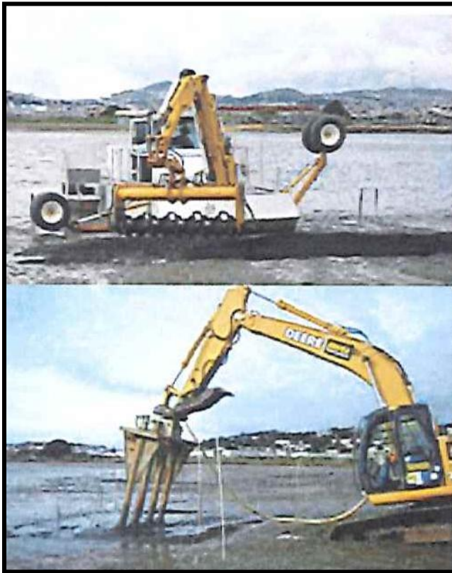
Figure 7-1 Pilot-scale Demonstrations of Activated Carbon Amendment Delivery into Sediment
