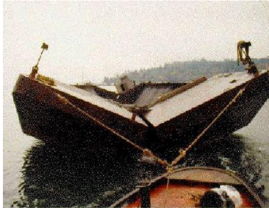
FIGURE 7-3 PLACEMENT OF THE IN-SITU CAP AT THE EAST EAGLE HARBOR OPERABLE UNIT, BAINBRIDGE ISLAND, WASHINGTON
